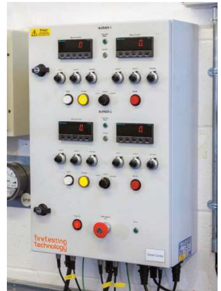
Gas control box mounted on wall
