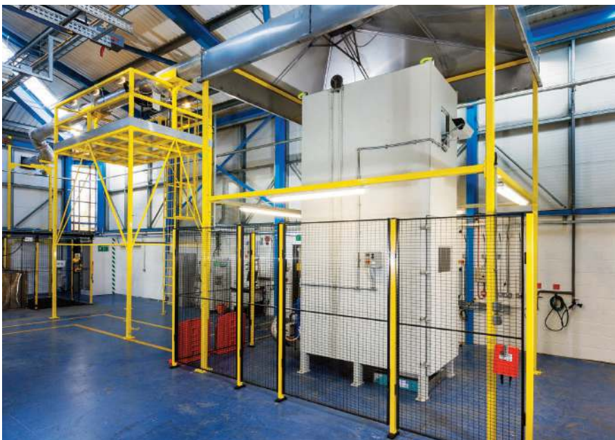
Side view of cable test chamber, hood and ducting
