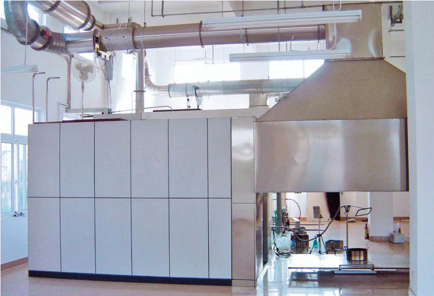
On-site system in a fire research institute
