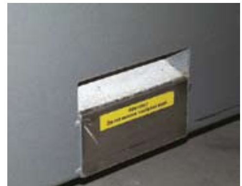
Emergency outlet for the safe draining of melt in case of crucible breakage
